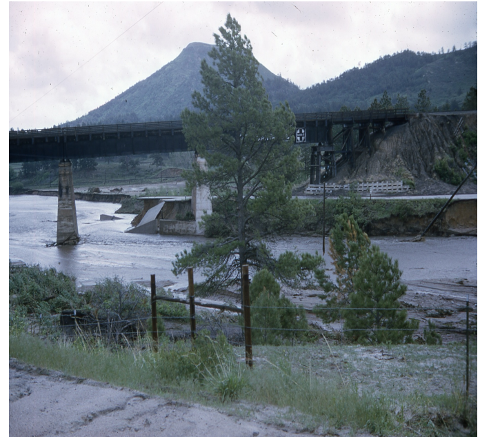
1965 flood picture of the railroad trestle at the south end of Larkspur
